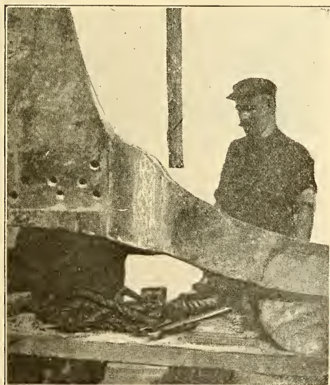
FIG. 50.—Weld on Sternpost of Tug No. 32, Made September, 1911.
